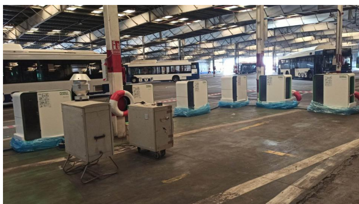
Figure 2. Illustration of CSIC measuring equipment and M+H air purifiers at AUVASA bus depot.
